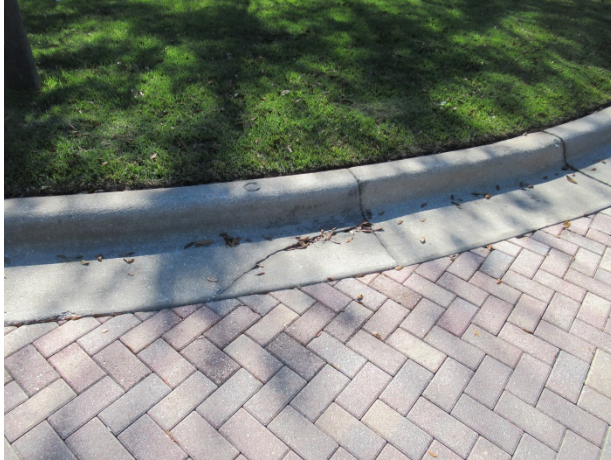
Minor concrete crack at curb and gutter
