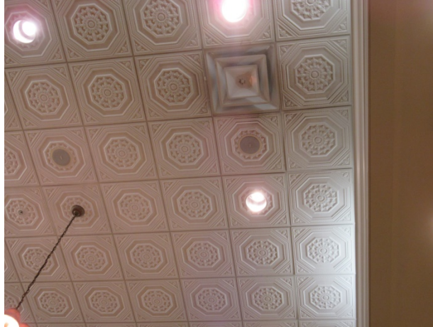
Acoustical ceiling tiles
