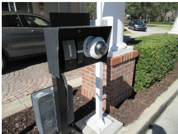
Main gate entry components
