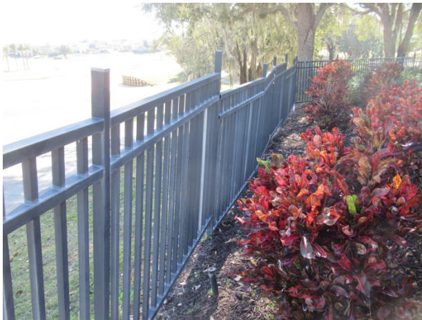
Leaning/loose section at Seven Eagles
