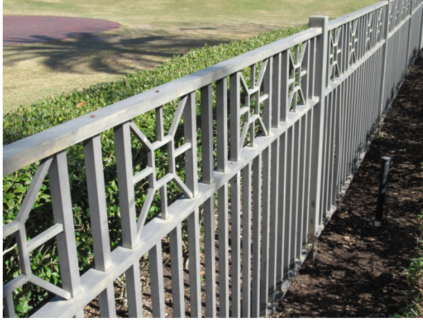
Typical aluminum fence, note fade
