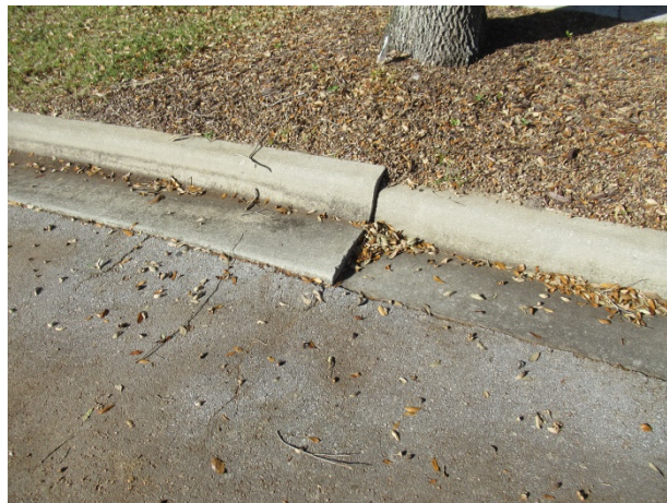
Settlement at curb and gutter
