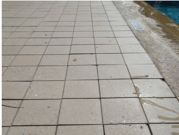
Spalls and minor settlement at Seven Eagles
