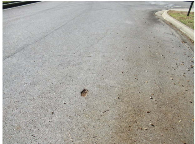
Example of minor damage
