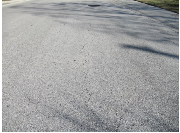
Minor cracks at Excitement Drive
