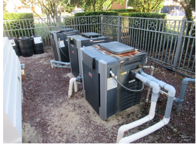
Rust at Carriage Point heater
