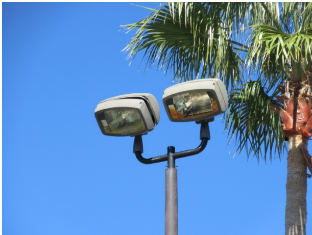
Loose fixture at Heritage B
