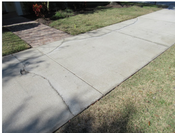
Multiple concrete sidewalk cracks near 1420 Reunion Boulevard
