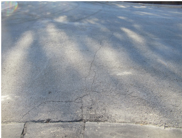
Minor cracks at Assembly Court
