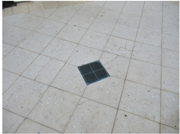
Cracked pavers at Carriage Point
