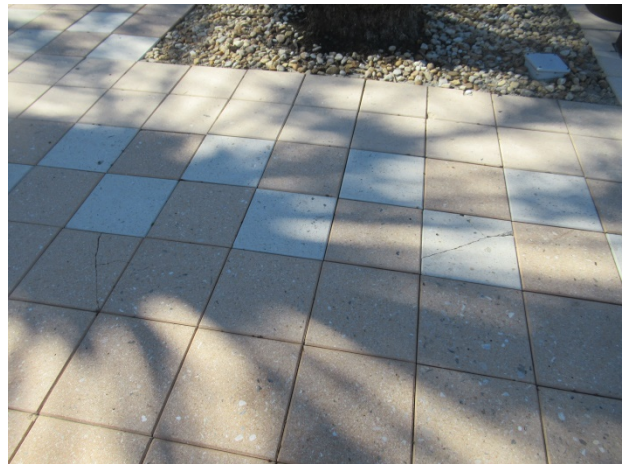
Isolated cracks at Seven Eagles
