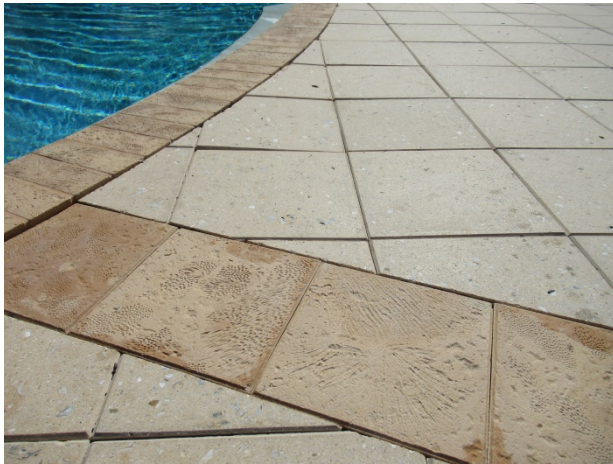
Minor paver lift at Heritage B
