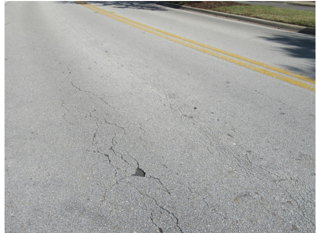
Cracks and deterioration at Reunion Boulevard
