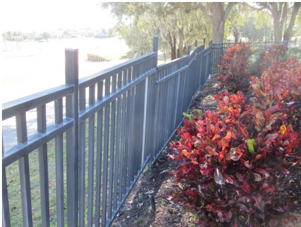
Leaning/loose section at Seven Eagles
