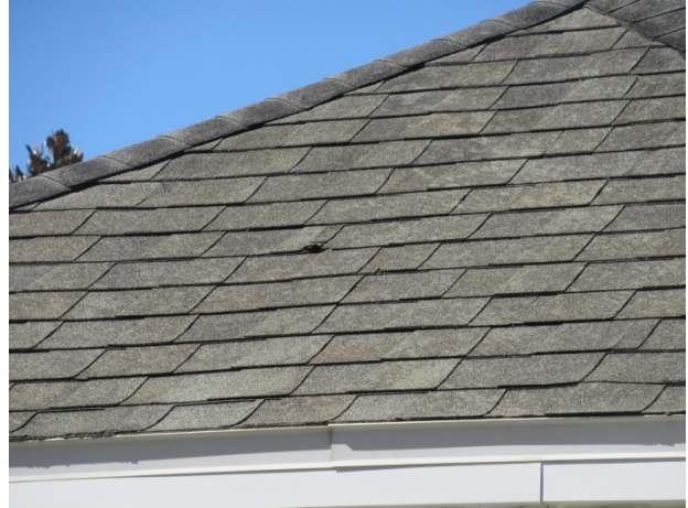
Shingle deterioration at Heritage B pool house
