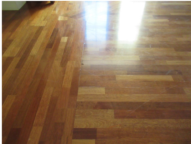
Minor deterioration at wood laminate floor
