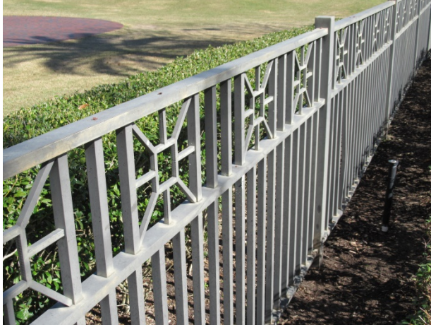
Typical aluminum fence, note fade
