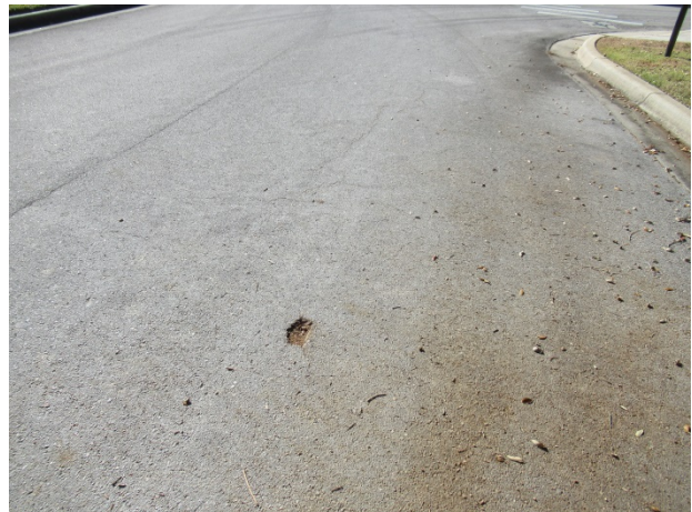
Example of minor damage
