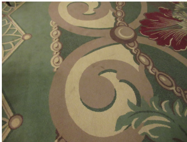
Minor stains at carpet
