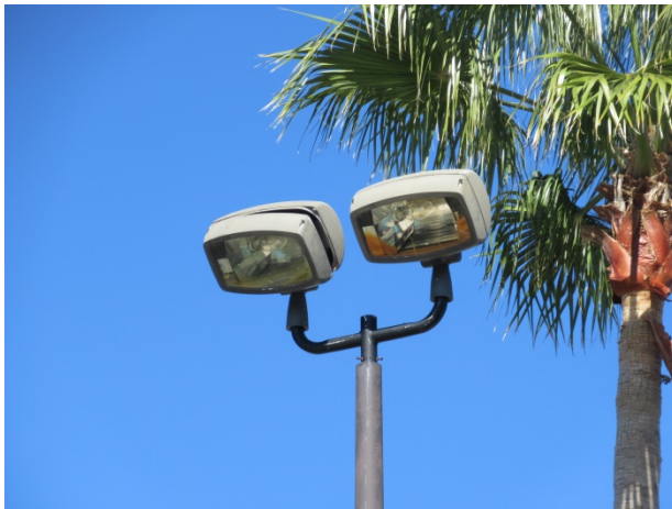
Loose fixture at Heritage B
