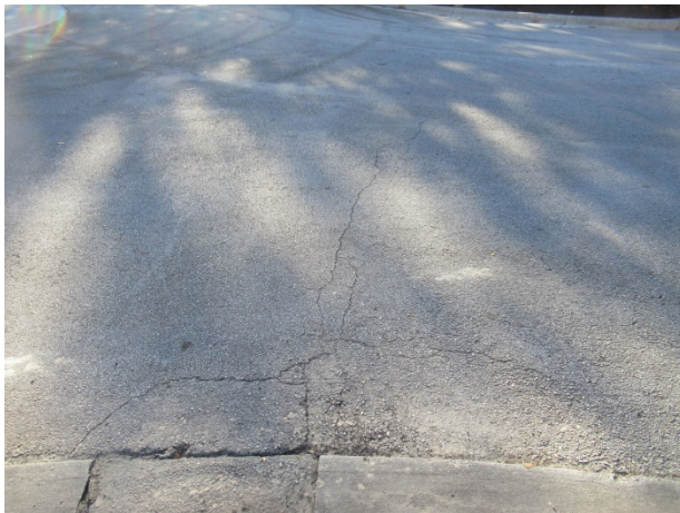
Minor cracks at Assembly Court
