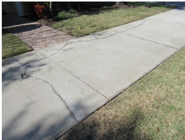
Multiple concrete sidewalk cracks near 1420 Reunion Boulevard
