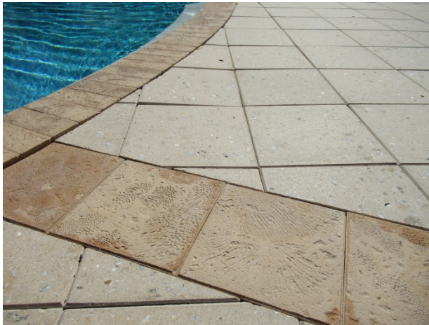
Minor paver lift at Heritage B
