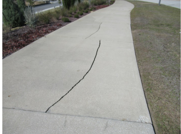
Sidewalk cracks near Tradition Boulevard gate house
