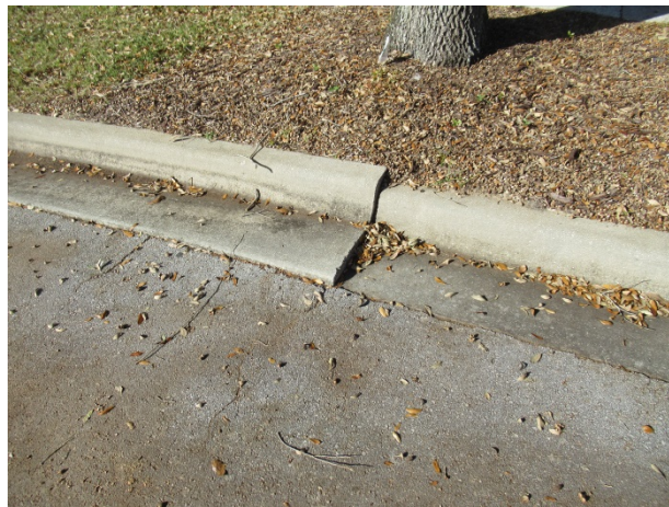
Settlement at curb and gutter
