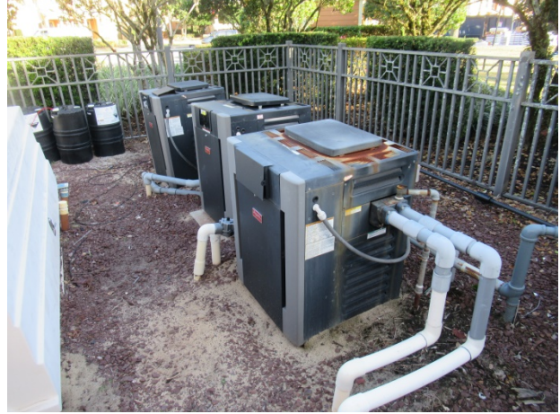
Rust at Carriage Point heater
