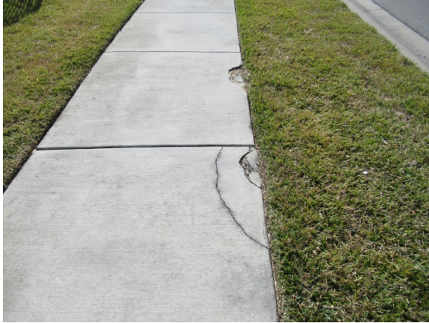
Concrete sidewalk cracks and damage
