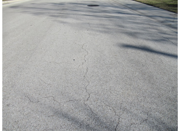
Minor cracks at Excitement Drive
